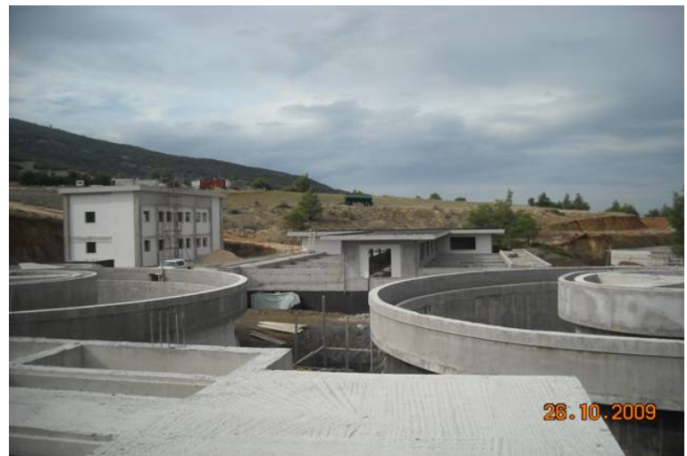
Patras Water Supply - Water Treatment Works
